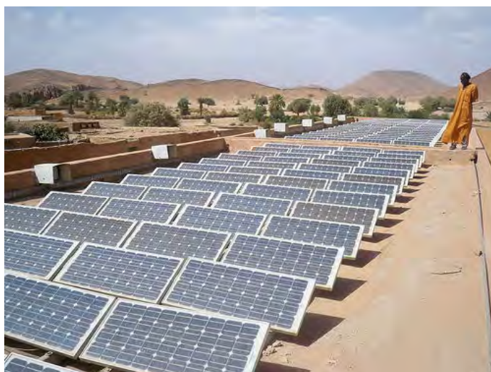
Solar panels on a rooftop. 1
